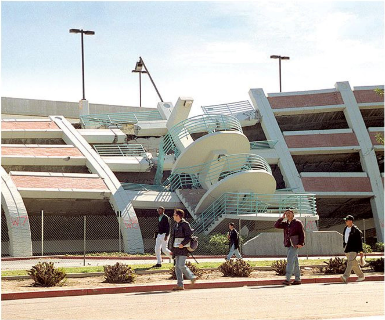
A hard-hit parking structure at Cal State Northridge. Photograph courtesy of Mark J. Terrill/AP Photo
