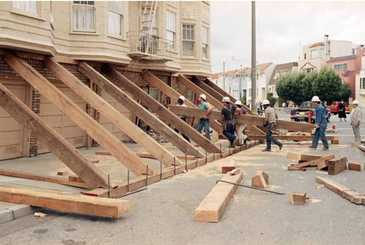
Workers shore up a soft-story building in San Francisco's Marina District after the Loma Prieta quake. San Francisco will now require owners to reinforce such buildings. (John Swart / Associated Press / October 23, 1989)
